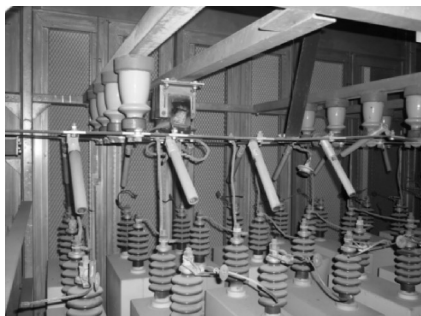
图1 整组外熔断器与不平衡电流互感器烧毁后 Fig. 1 Entire set of external fuses and unbalanced current transformers burned
